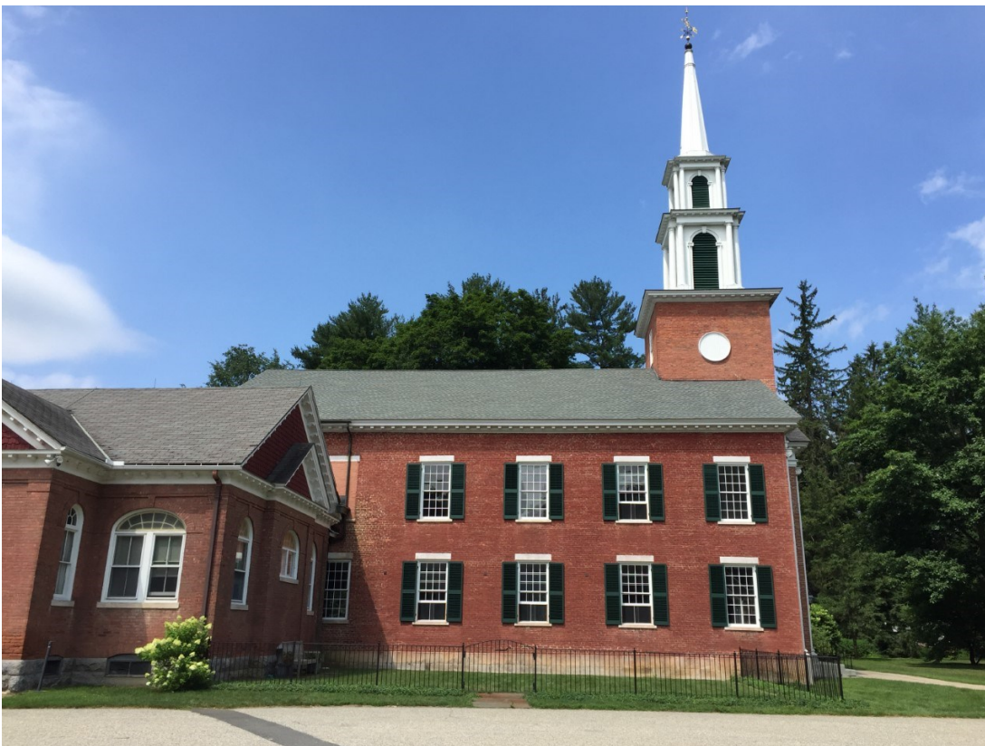
Contractor Don Hayward recently installed the beautifully restored shutters on the east side of the sanctuary.
