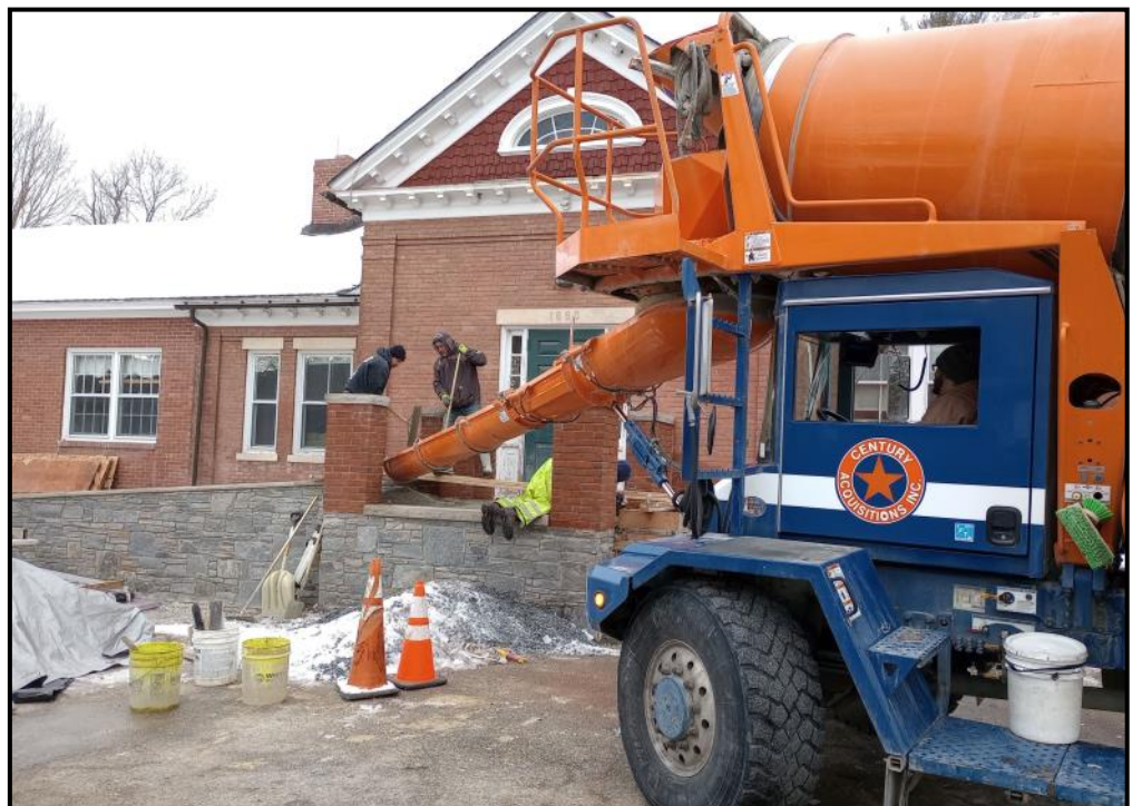
Another hard-working crew. John's Excavating finished pouring the concrete ramp and steps on December 19. Cold work! They poured around high-tech heating wires that melt snow and ice.
